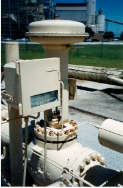
Figure 7.a - Before —Power plant regulator with typical controller installed on a globe valve with spring & diaphragm actuator. Constant cycling of control valve and constant bleed to atmosphere. The system required a valve positioner.
