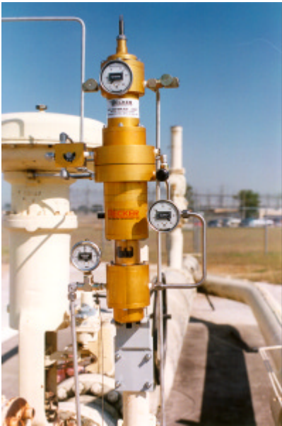
Figure 7.b - After —Power plant regulator retrofit with Becker VRP-SB-PID Controller on same control valve and actuator. Stable pressure control to power plant with ZERO atmospheric bleed in steady state. The need for a valve positioner was eliminated.
